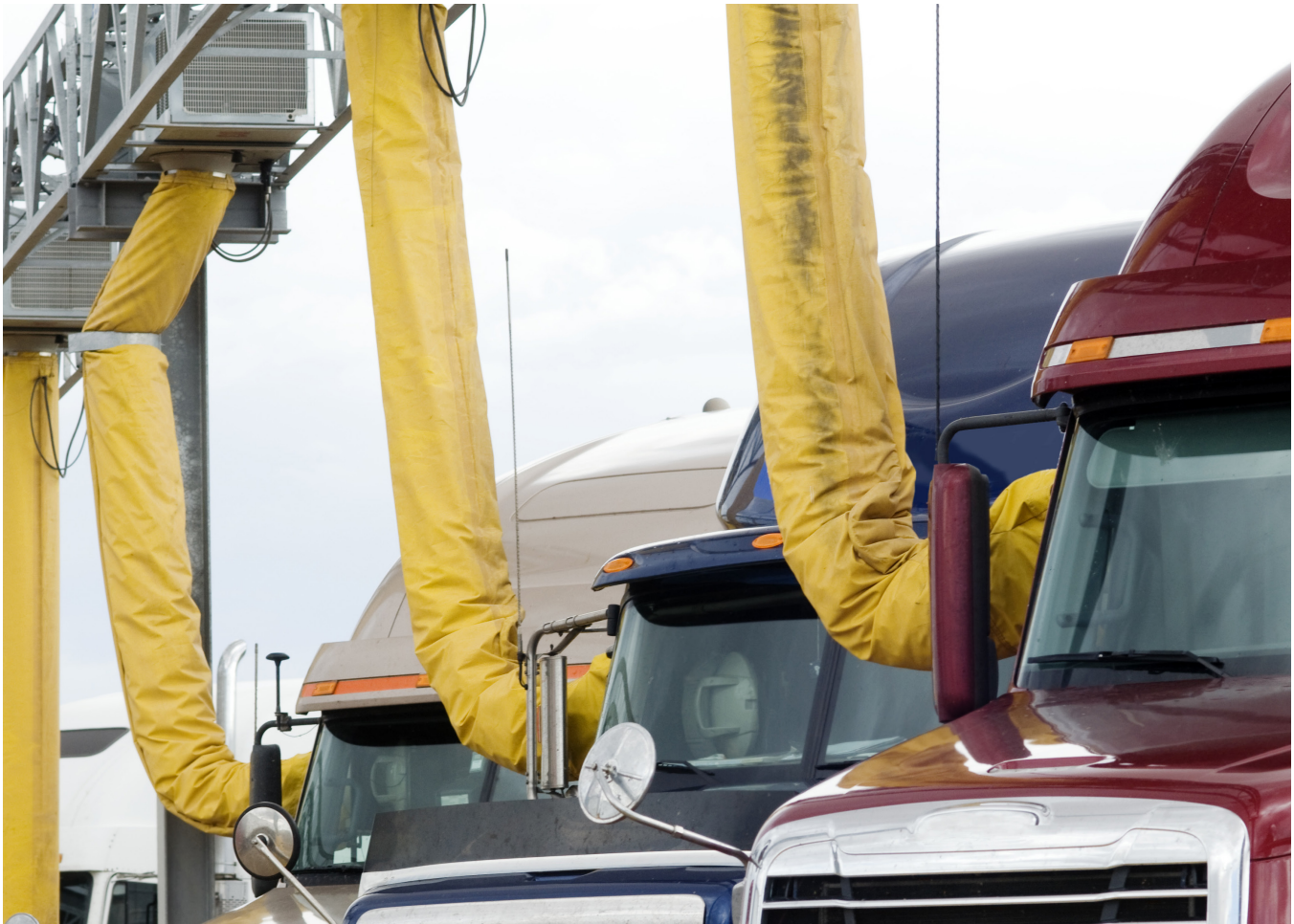
Example of a Truck Stop Electrification installation (an auxiliary HVAC unit) to reduce truck idling for cooling/heating.
